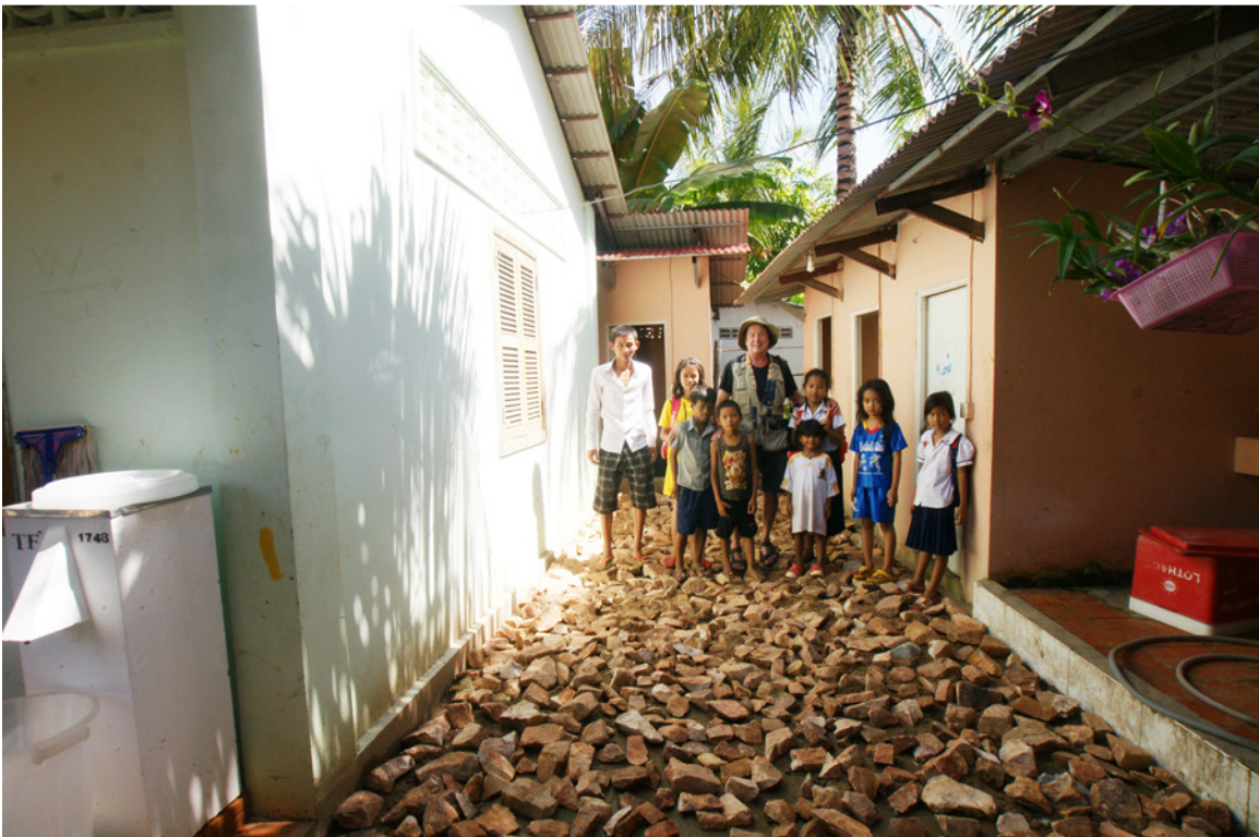
Cambodia Orphanage, installing rock for the foundation for the new patio floor.
